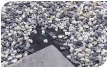
Too little aggregate
